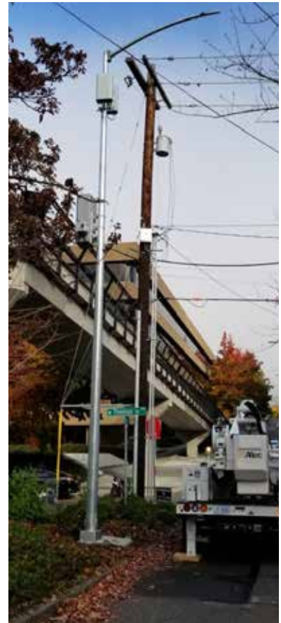
Image 4: Metal pole with side-mount panel antennas and equipment cabinet
