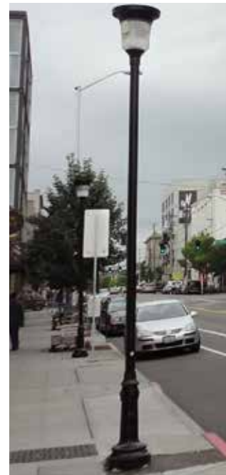
Image 6: Light pole with post-top light
